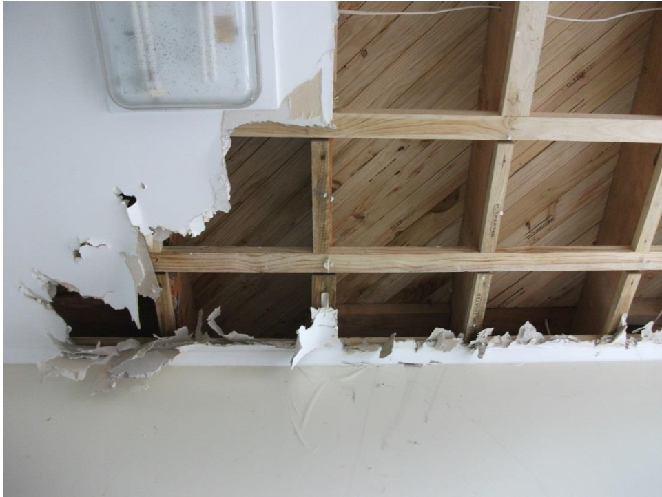
Figure 6 - First Floor Diaphragm at the Interface between the End and Central Portions
