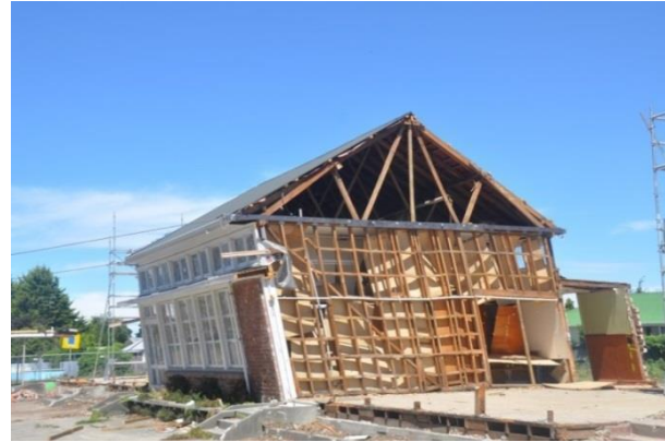
Figure 7. Building showing high levels of drift during the transverse test
